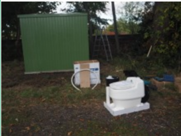
The new loo being fitted. Don't worry - the toilet goes inside the green building!
